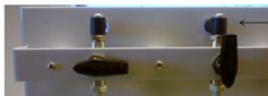
Valves in vent position and in draw sample position.
